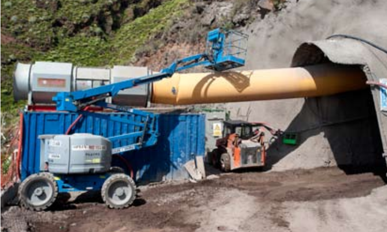
Construction begins on the tunnel that will carry the water down from the upper reservoir
